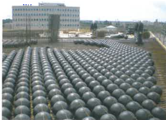
Fig. 1. Installed Cobiax Eco-Line system void formers before installing the upper reinforcement layer and concreting (erection of an office building in Bremen)
